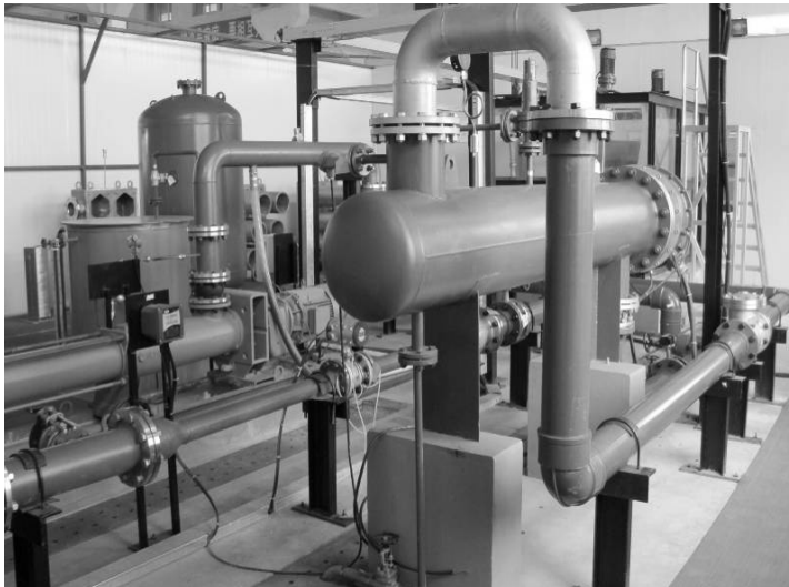
Fig. 5. Photograph 1 of the test system (containment sump strainers)
